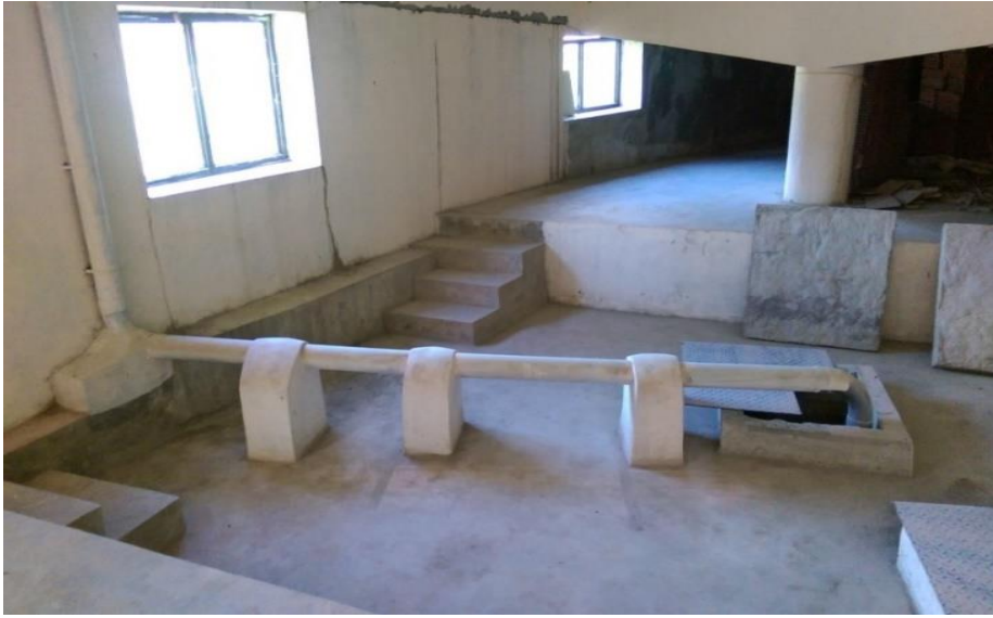
Fig.3. Recharge well. Rainwater collected from rooftop after filtration is recharged into an open well
