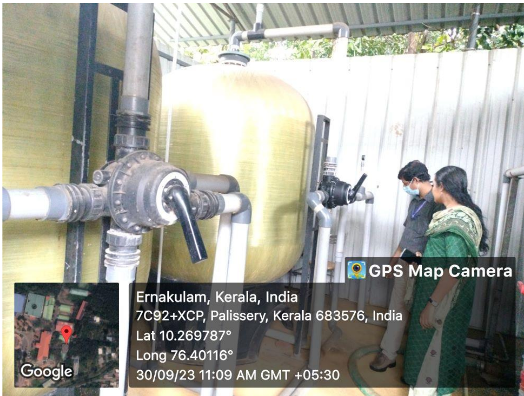
Fig. 4 Drinking Water Treatment Plant
