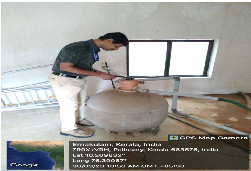
Fig. 2 Bore well recharge installation. Rain water collected at rooftop is treated using Pressure sand filter before taken for bore well recharge
